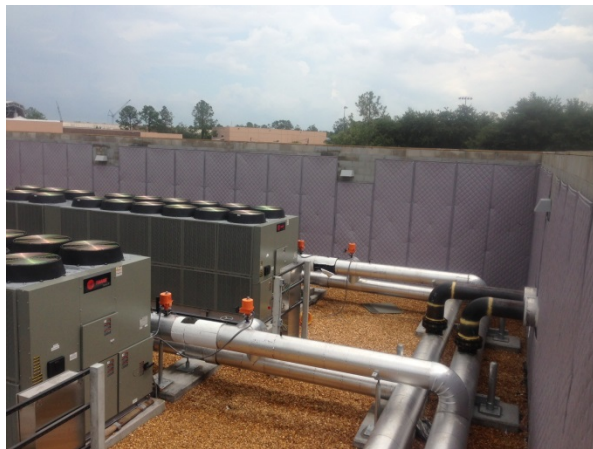
CMU block wall enclosure with HUSH FLEX™ exterior grade curtain panels.
