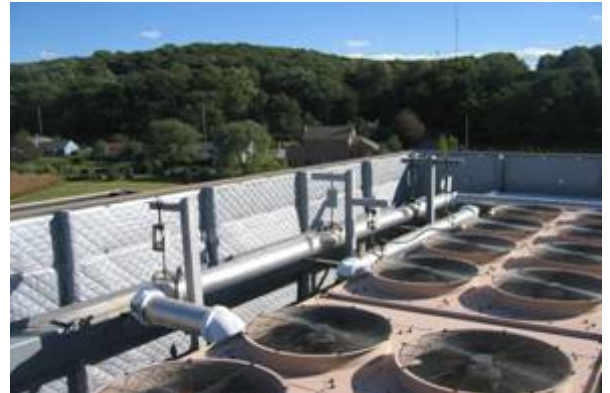
HUSH FLEX™ curtain panels attached to inside of existing non-acoustical metal screen walls.
