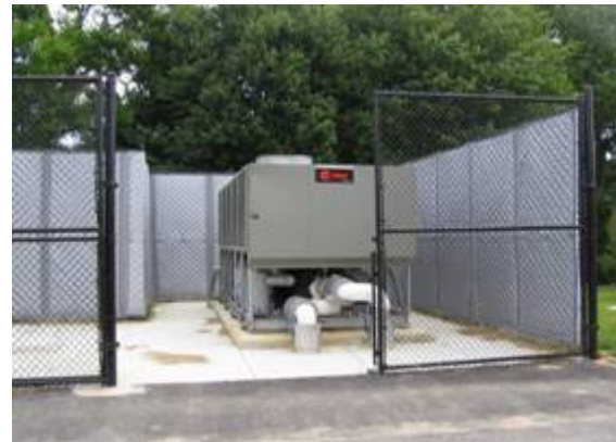
Air-cooled screw chiller with HUSH FLEX™ curtain panels attached to chain link fence.
