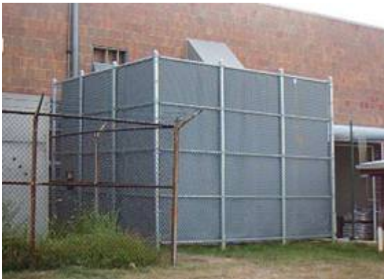
Cooling tower curtain system attached to chain link fence.
