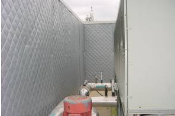
Concrete/stucco wall structure with HUSH FLEX™ panels creates efficient chiller sound enclosure.
