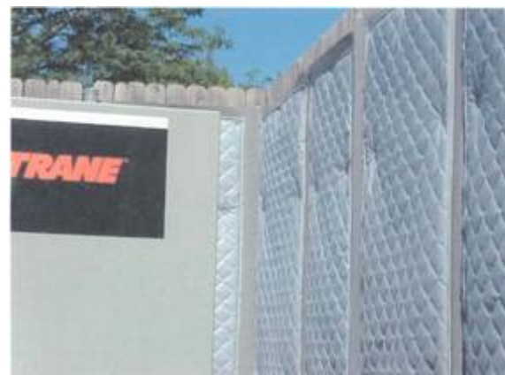
Close-up of HUSH FLEX™ panels on inside of wood slat fence enclosure.
