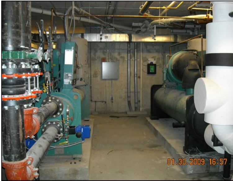
Untreated Screw Chiller
