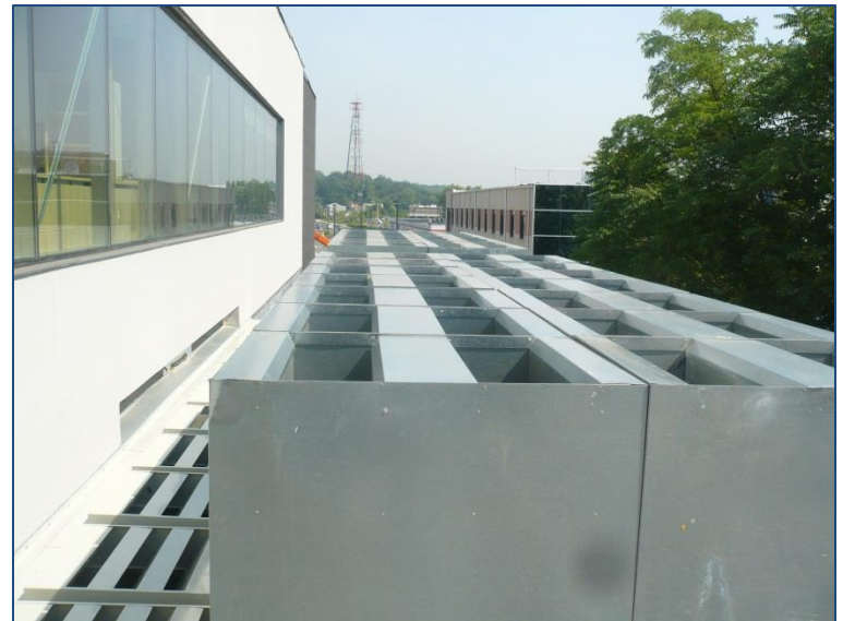
Condenser Fan Discharge Stack with Silencers
