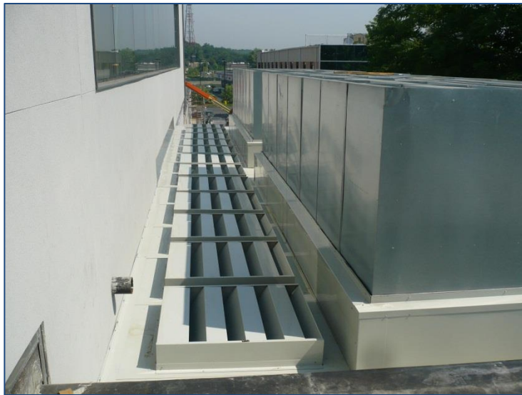
Roof Mounted Air Intake Silencers
