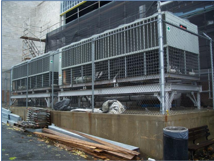
Untreated 200 ton screw chillers
