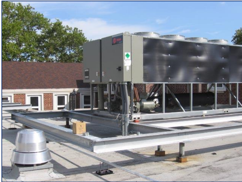
Oversized Chiller Dunnage Support Frame
