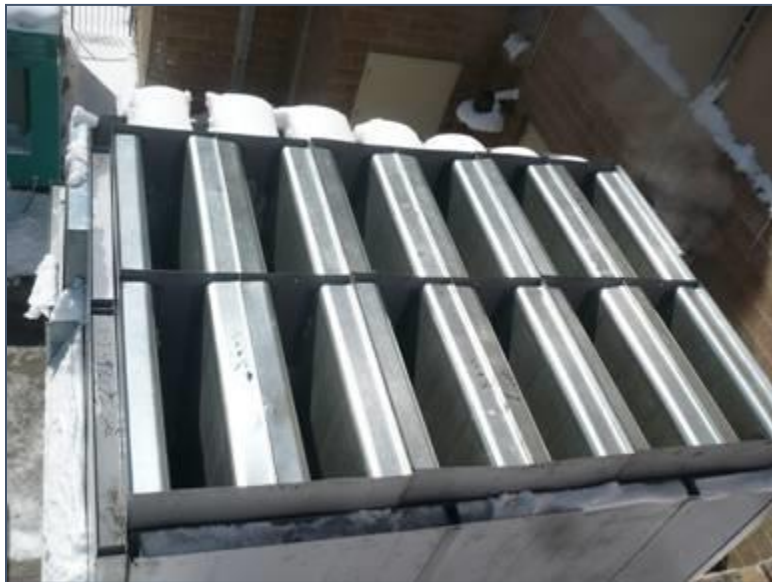
Top View Fan Discharge Silencer Bank
