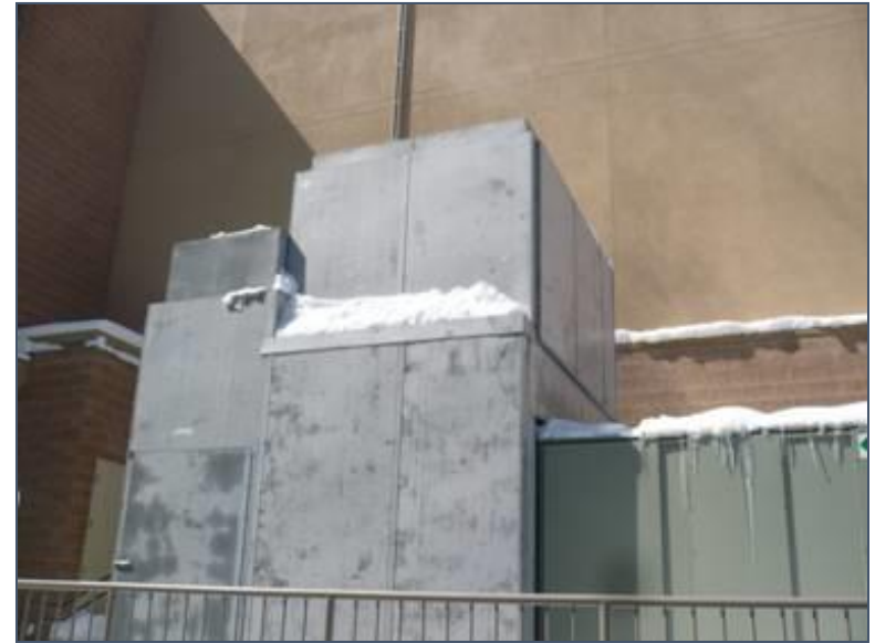
Intake & Discharge Silencer Banks
