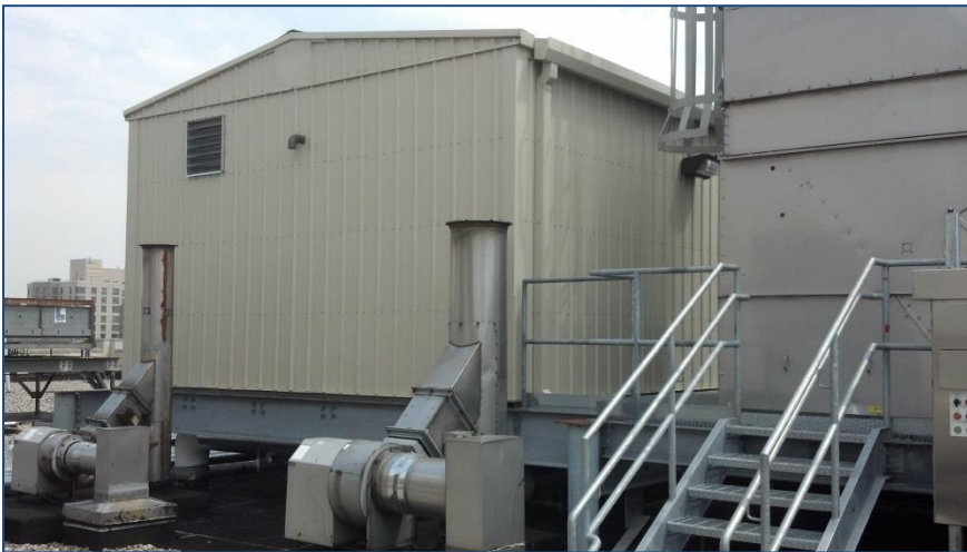
Enclosure Access Stairs
