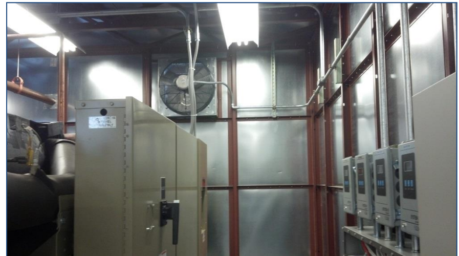
Screw Chiller & Controls Inside Enclosure
