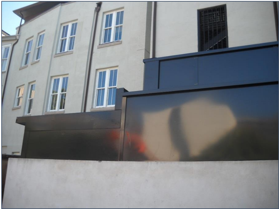
Ultimate™ System Roof Discharge Stack with Condominium Windows in Background
