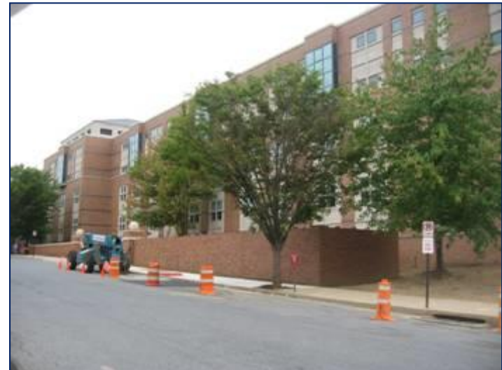
Chiller Enclosure Seen From Street. Chiller pit floor elevation is 5' below surrounding grade to control overall wall height.
