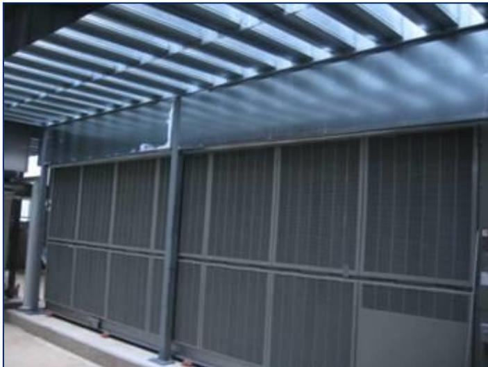
Roof Mounted Air Intake Silencer Banks Seen From Inside
