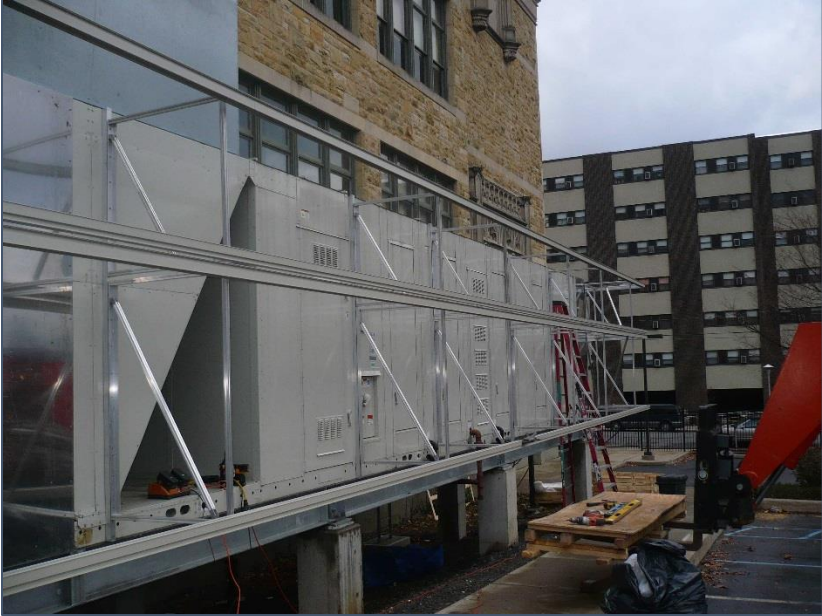
Aaon Unit with Unit Supported Screen Framing
