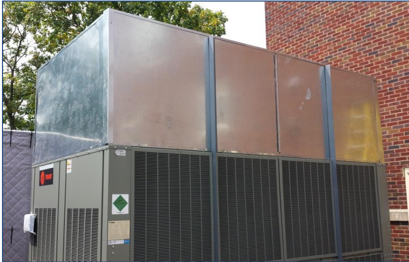
Close-Up of Top Mounted Unitary™ System Discharge Silencer Stack
