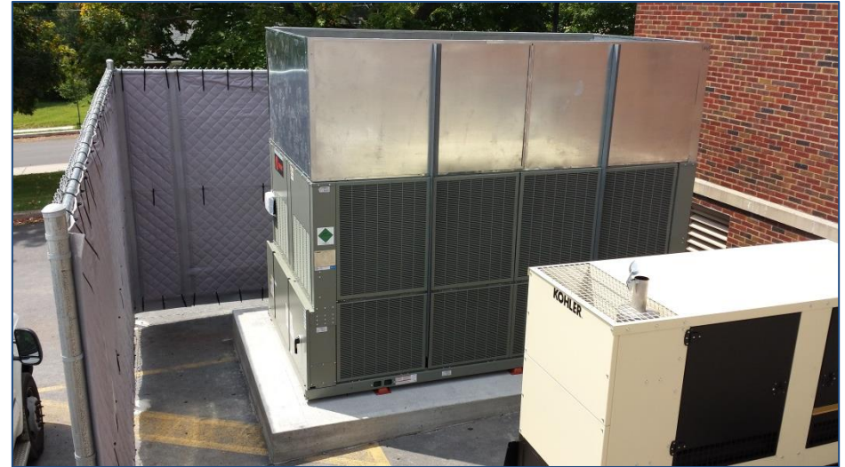
Inside View of Premium™ “TS” System Enclosure
