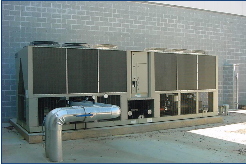
Untreated Screw Chiller
