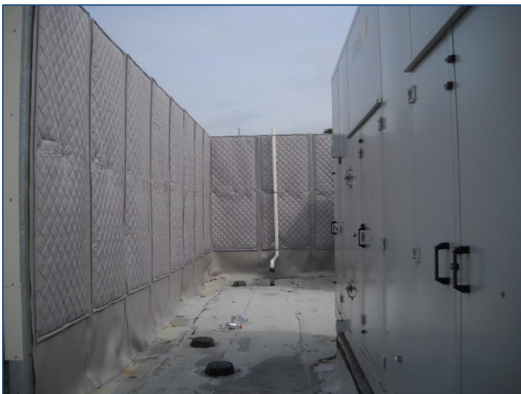
Inside View of Finished Premium™ “OF” System
