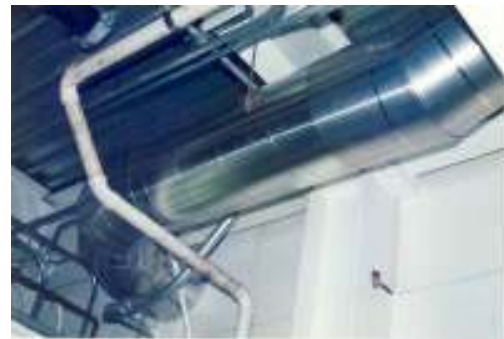
Dust collector material transfer ducting treated with LVAL-100 and HUSH BATT™ HB-200 insulation.
