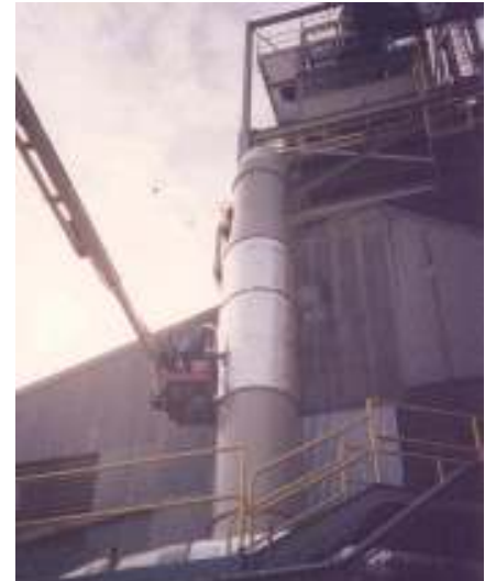
Installation of HUSH WRAP™ LVQ-110-LAG composite material on outdoor industrial exhaust ducts.
