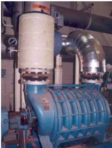
Installation of built-up system using HB-400 HUSH BATT™ insulation covered with type LVAL-100 barrier. HUSH SEALANT™ acoustical sealant, HUSH COVER™ removable covers and HUSH BLOCK™ type LM (loaded mastic) materials are all part of HUSH WRAP™ built-up systems.
