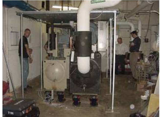
Screw chiller on type AB System next to school NC-20 auditorium.
