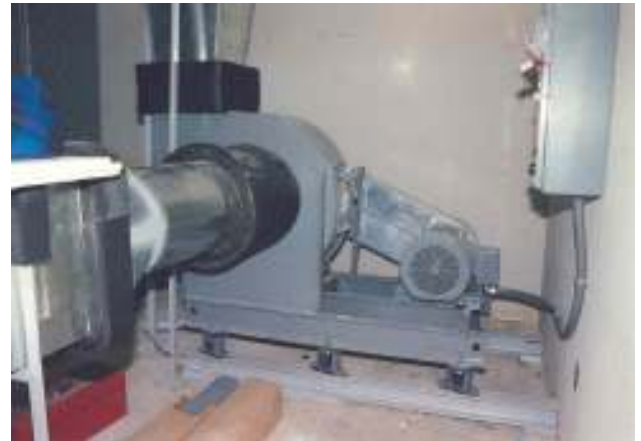
HVAC ventilation fan on structural base with type HS isolators.
