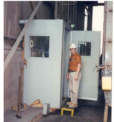
Custom modification of a model HGSO-2 at a cement plant.
