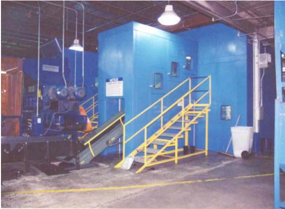
Grinder enclosure using HUSH GUARD™ HG-400-SC panels. Scrap feed conveyor requires a separate feed tunnel complete with access doors to meet the 85 dBA requirement.
