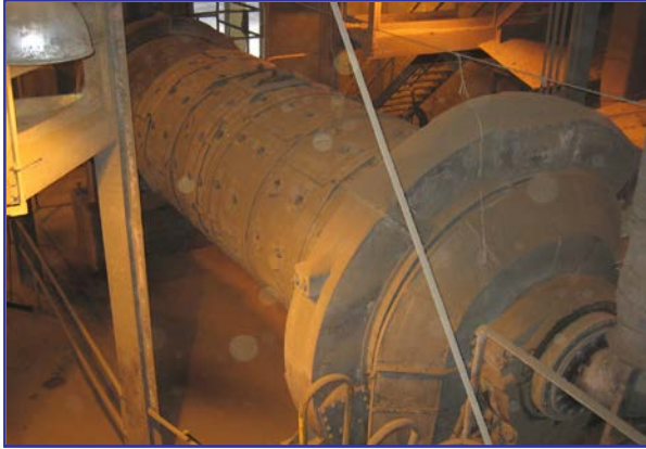
Ball Mill Wrap with exposed liner bolts at a cement plant.
