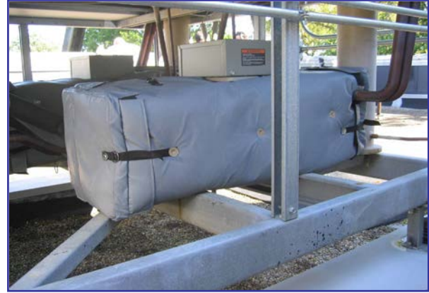
HUSH COVER™ Model HC-500S-1" blankets for air cooled screw chiller compressors.
