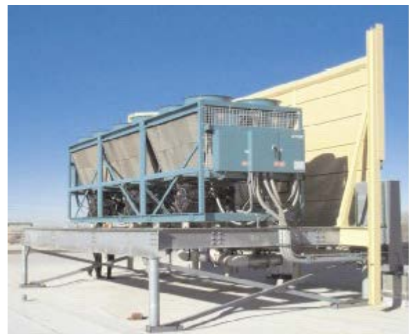
Air-Cooled Chiller with Direct Path barrier wall to block and absorb noise generated by the condenser fans and compressor circuits.
